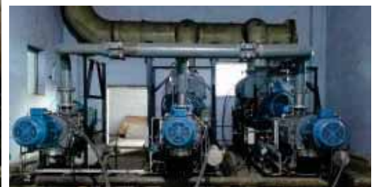
VD Pump house
