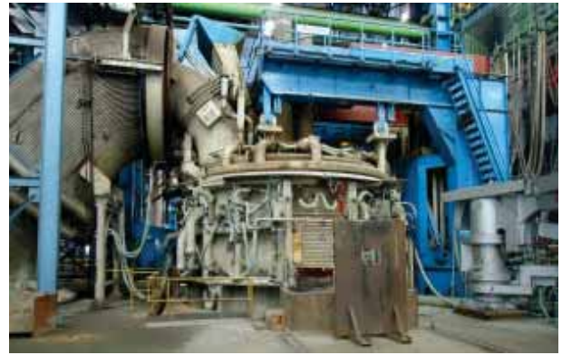
100T EAF, Monnet Ispat & Energy Ltd., Raigarh, India
