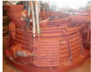
LADLE FURNACE ROOF
