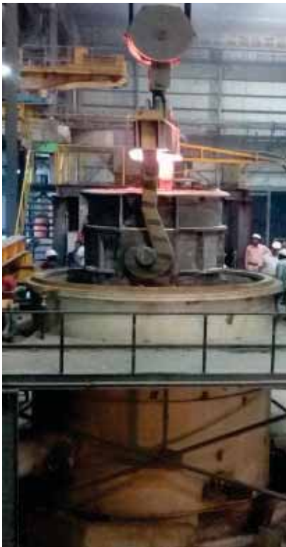
VD Hot commissioning
